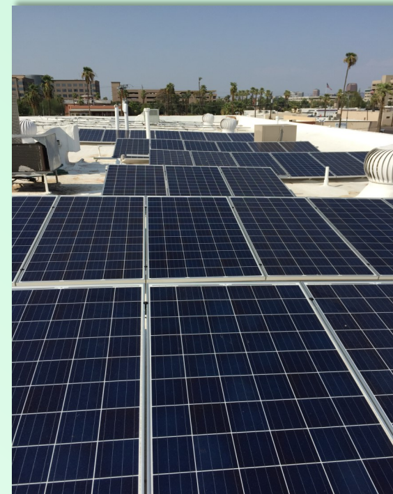
Solar panels covering entire roof
