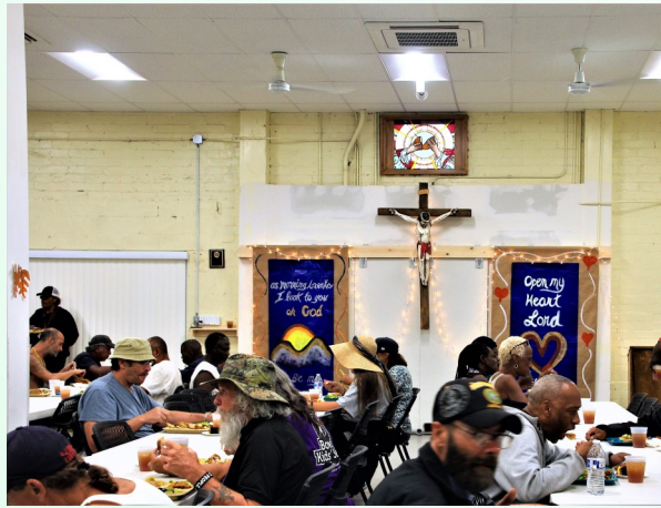
new dropped ceiling and lighting fixtures on south side of dining room
